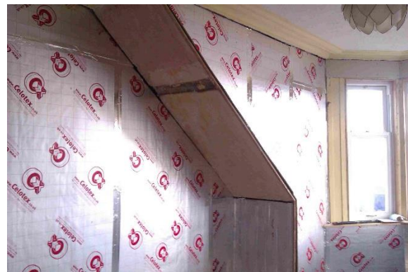
Figure 5.2 Insulation and studs covered with second 12 mm sheet insulation prior to installing foil backed plasterboard
